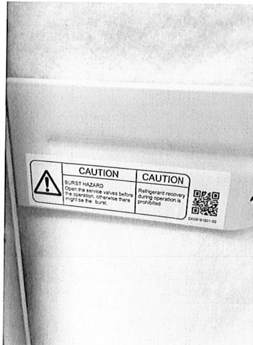
WARNING/CAUTION Label near Compressor
